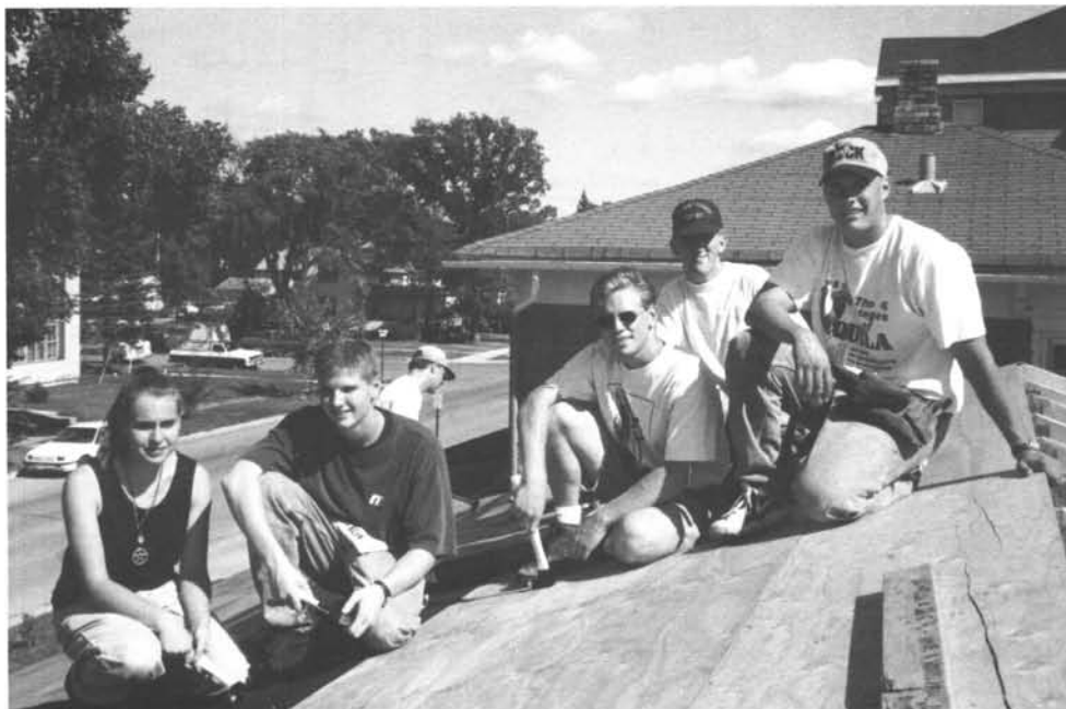
Students aspire to new heights (or staying on top) while helping roof the Crookston Habitat for Humanity house.
