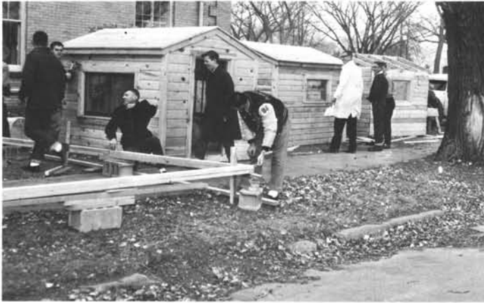
Two of the projects undertaken by the carpentry classes this year are building a garage and playhouses.
